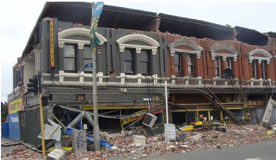
Figure 2. Collapse of verandah due to out of plane failure of brick wall.
