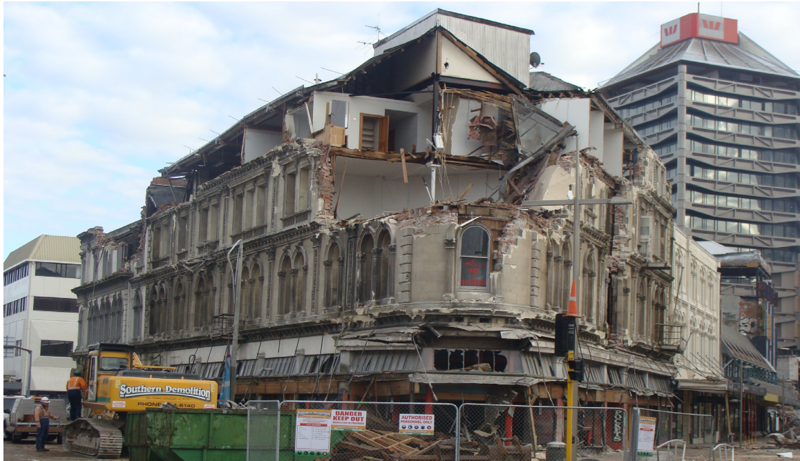
Figure 1. Face loading failure of unreinforced masonry (URM) walls.
